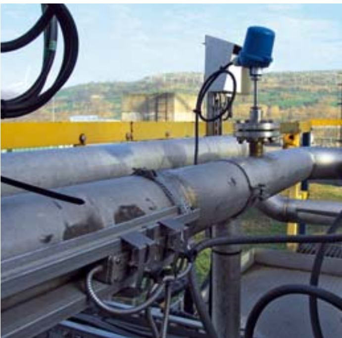
Measuring point at the filling station for nitric acid
